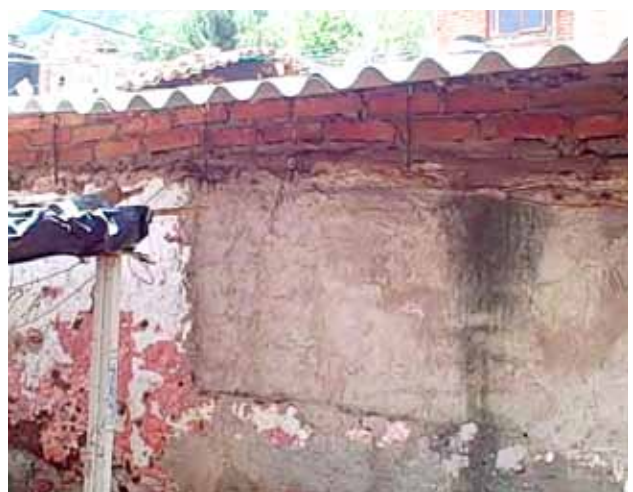
(roof from outside): The roof hanging over into the front 'patio' area. To put the roof on, it was necessary to do brickwork along the front of the house.
