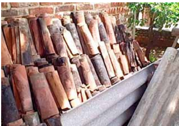
(tejas we removed): Before we could begin installing the roof, we had to remove the existing one, a mix of the roof tiles you see here and reeds tied to wooden beams.
